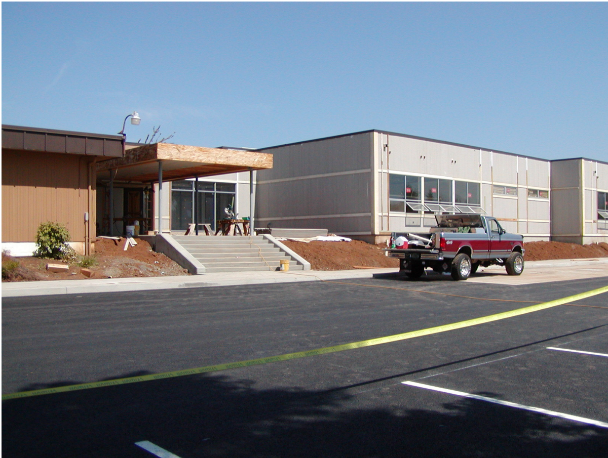
Although work is still underway on the remodeling of Lacombe School in this August 2002 picture, the new look of the school is obvious.
